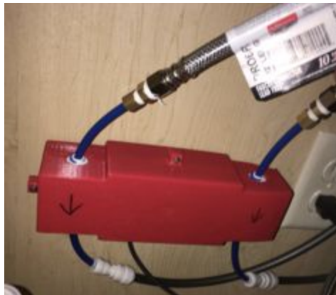
Figure 7: Installed Flowmeter Sensor
